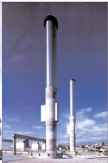
Fume Extraction Chimney
